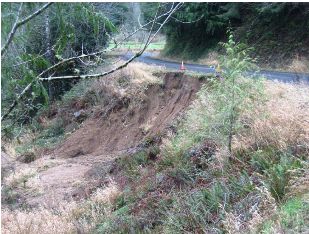
Figure 4.9. Road related mass wasting.
