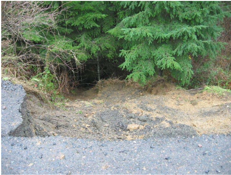
Figure 4.11. Road related landslide, moving downstream.
